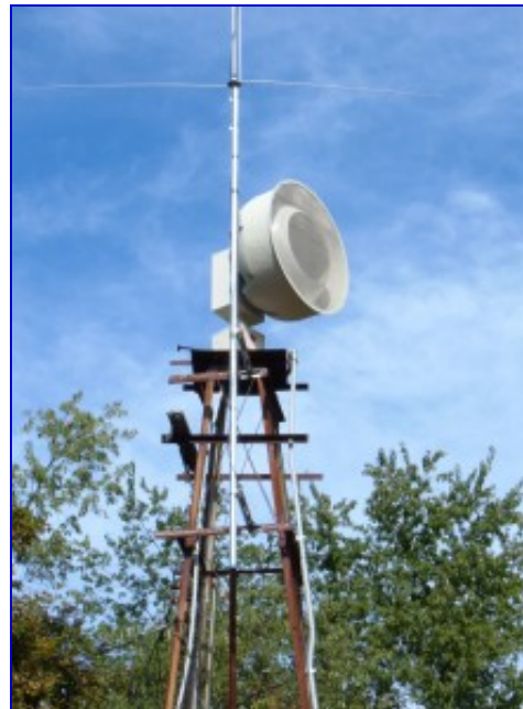
New siren installed in the Town of Tioga (Photo: Rick Stilson)
